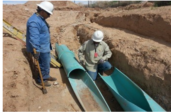
Pipe had to be cut past the extent of the traveled crack to be properly repaired Image Credit: Chris Augster, UA Local 412
