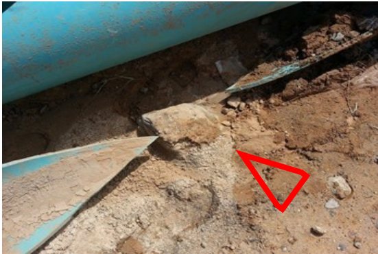
Rock left in soil bed did catastrophic damage to this pipe Image Credits: Chris Augster, UA Local 412
