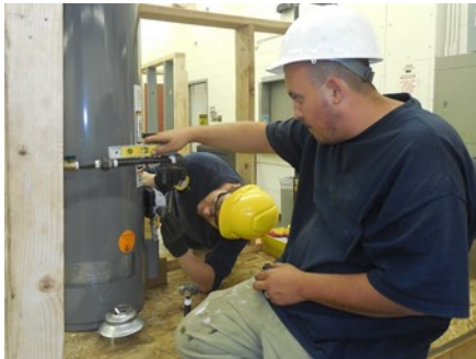
Mr. Thomas Hulse checks the level of the gas line that is hard piped to the water heater
